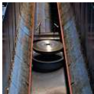
Milling the clamped plate edges provides an optimum preparation for the welding process
